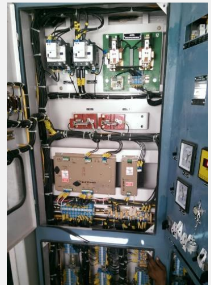
LCC107B in Control Cabinet
